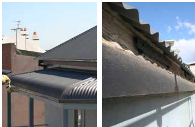
Villa Franca, 2 Scott St Currently Fitted with Gutter Grip®
